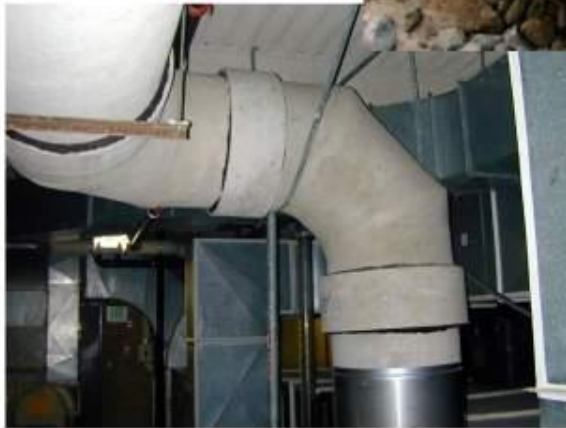
ASBESTOS CEMENT LAB FUME HOOD EXHAUST DUCT
