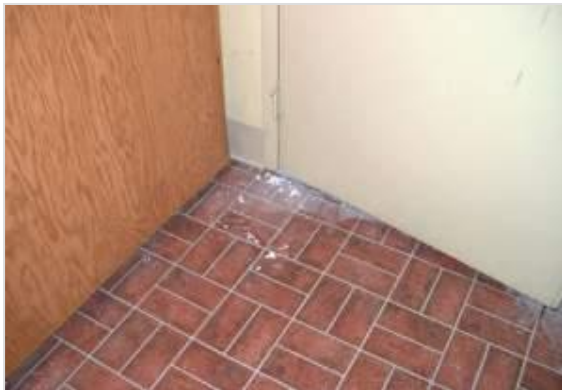
Asbestos debris on floor
