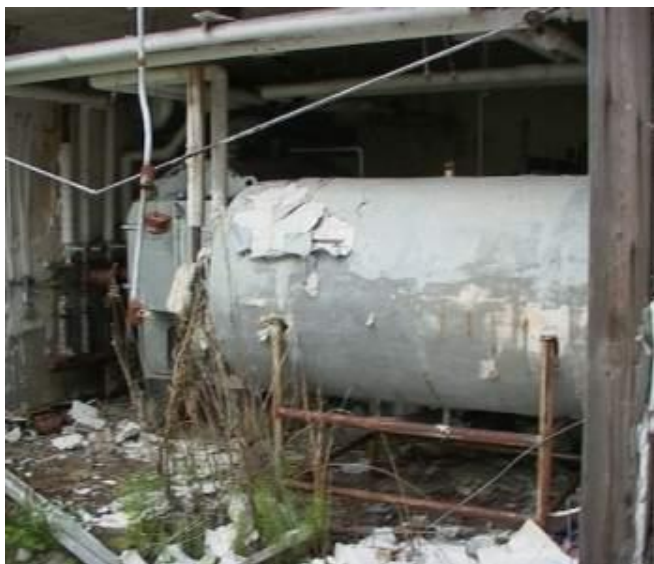
Asbestos insulated boiler
