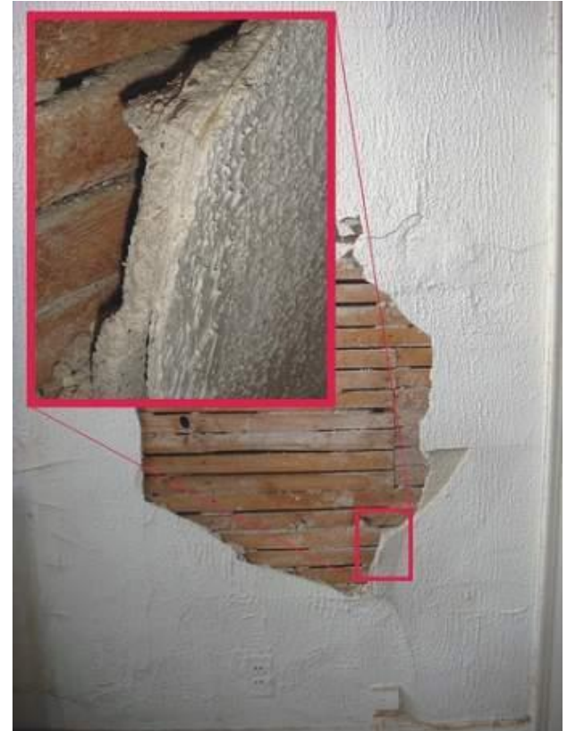
Plaster with asbestos
