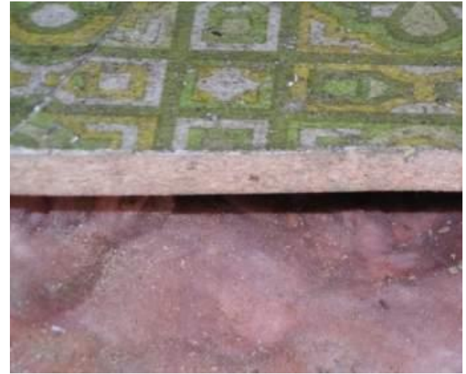
Sheet vinyl containing asbestos
