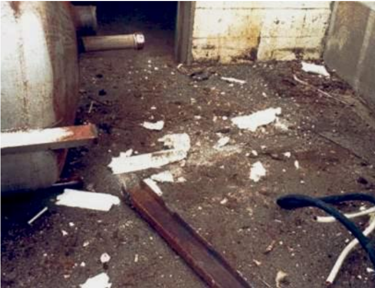
Loose asbestos debris from demolition project
