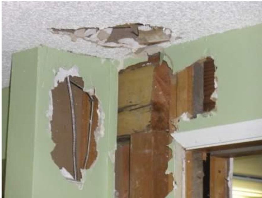
Damaged ceiling material
