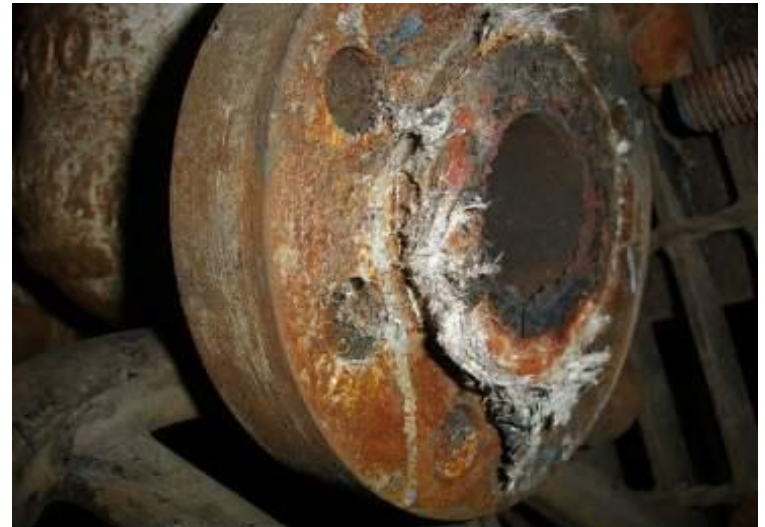
Damaged asbestos gasket
