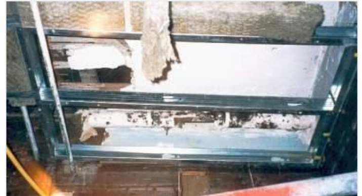
Damaged asbestos pipe insulation
