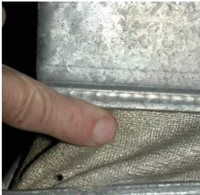
Asbestos fabric in HVAC system
