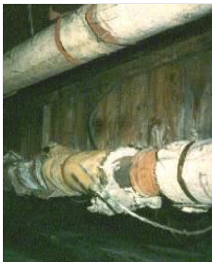
Asbestos insulated pipe
